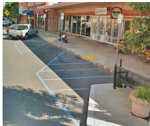
Accessible parking space with access aisles on both sides located on North Market Street in Wailuku.
